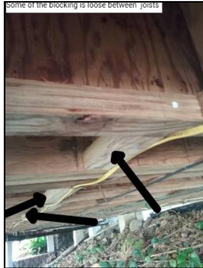
Some of the blocking is loose between joists
